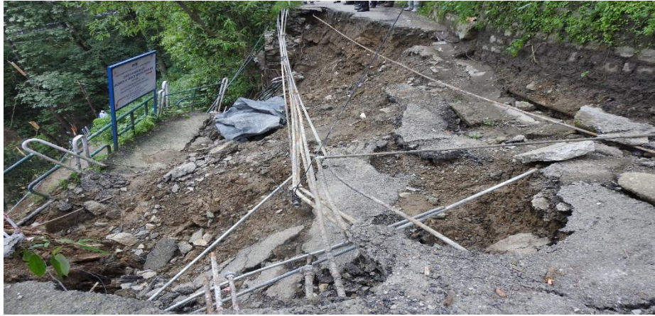
Figure 8 Footpath landslide at Himland, Shimla, district Shimla, Himachal Pradesh
