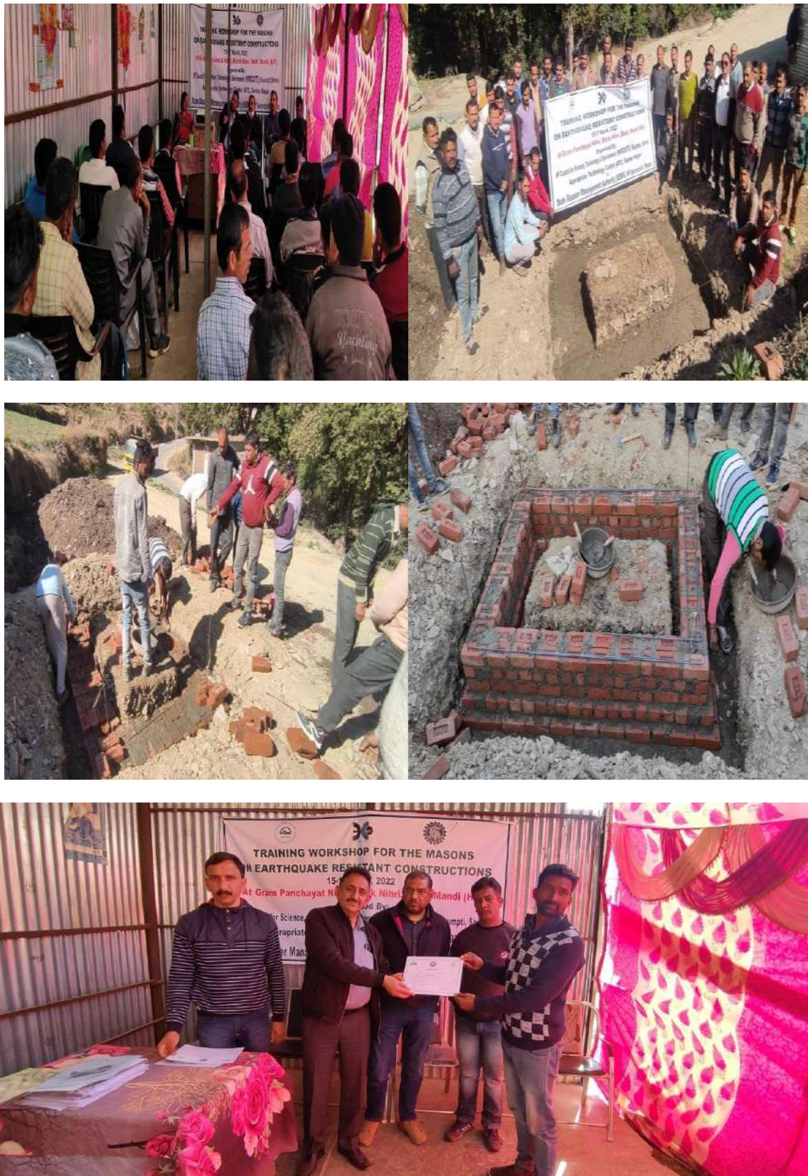
Figure 22 Certificate distribution to masons during 3 days training programme at Gram Panchayat Nihri, district Mandi
